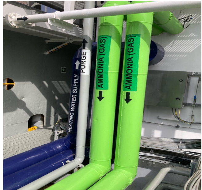
Ammonia pipes aboard the Green Pioneer, the world's first dual-fueled ammonia- and diesel-powered ship. See case study in Section IV for more details. (Photo source: Michael S. Lerner/Energy Vision.)
