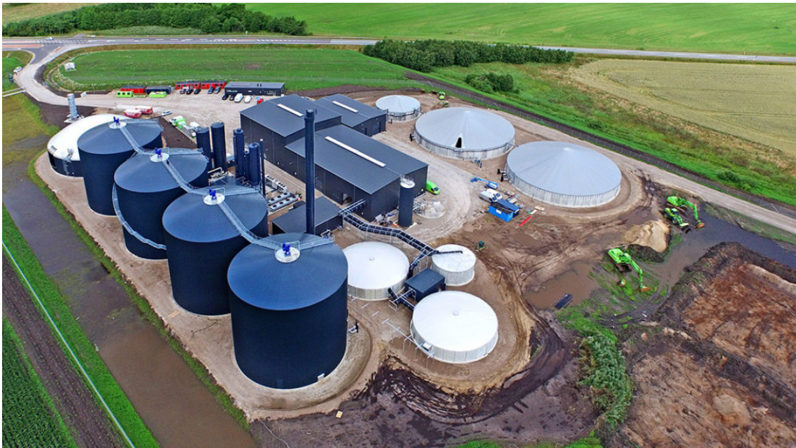
Nature Energy anaerobic digestion facility produces RNG from livestock manure and source separated organics.
