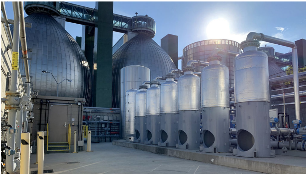
Newtown Creek water resource recovery facility in Brooklyn, NY is gearing up to process 500 tons/day of food waste. Photos courtesy of Energy Vision
