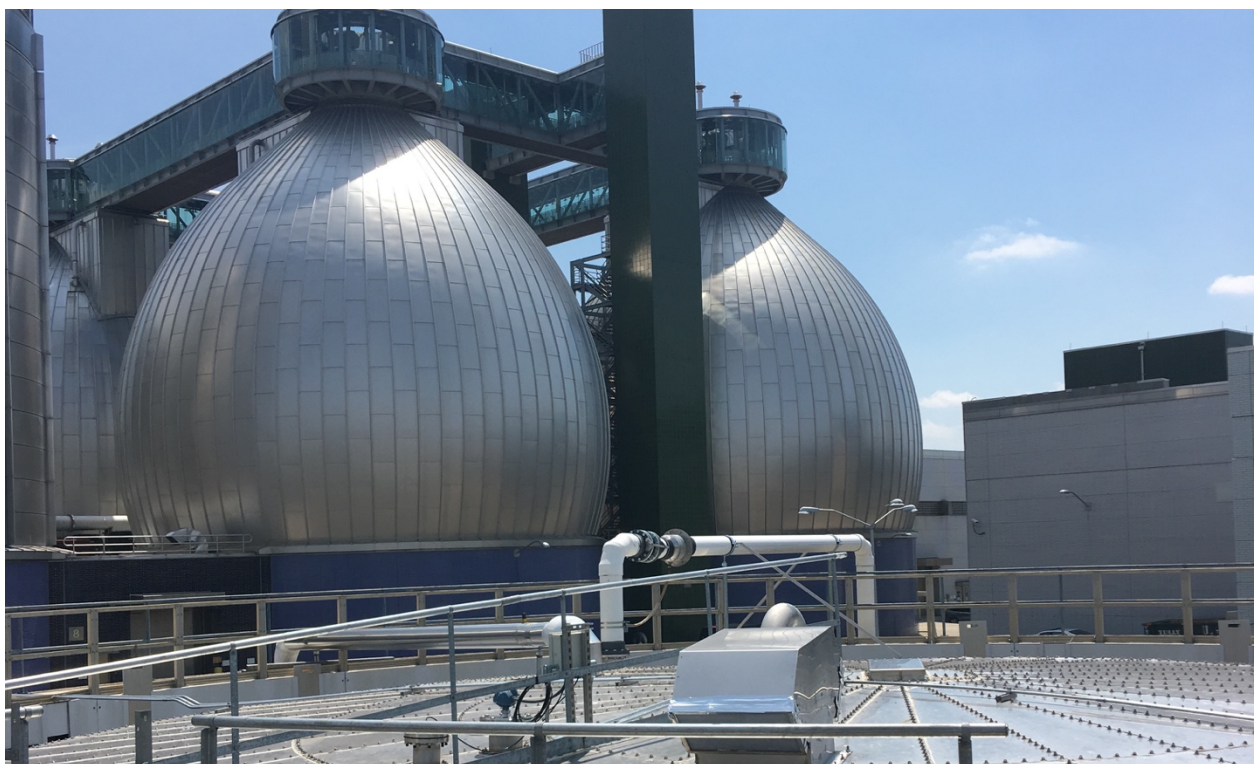
The Newton Creek municipal solid waste digester in Brooklyn, New York. Image courtesy of Energy Vision.
