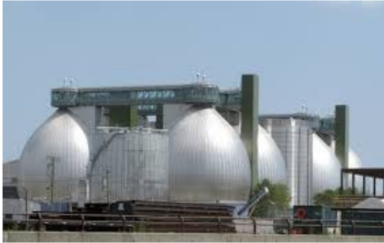
Newtown Creek Anaerobic Digesters in Green Point, Brooklyn. Credit NYC DEP.
