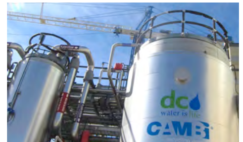
One of the tanks at DC Water's advanced wastewater treatment facility
